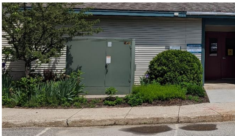
Figure 15 6 Spruce St. Electrical Distribution Transformer
